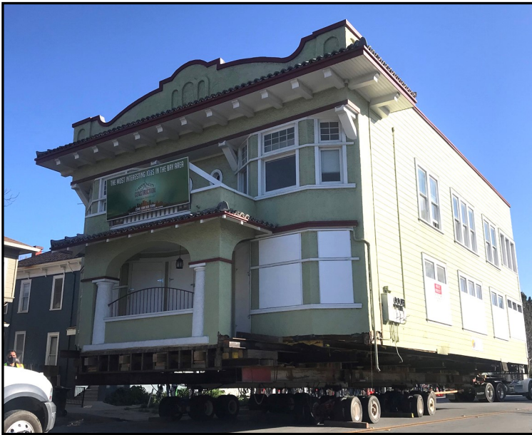
The Pallesen, sitting on 40 rubber tires, slowly crawling down E. Reed Street to its new home.
