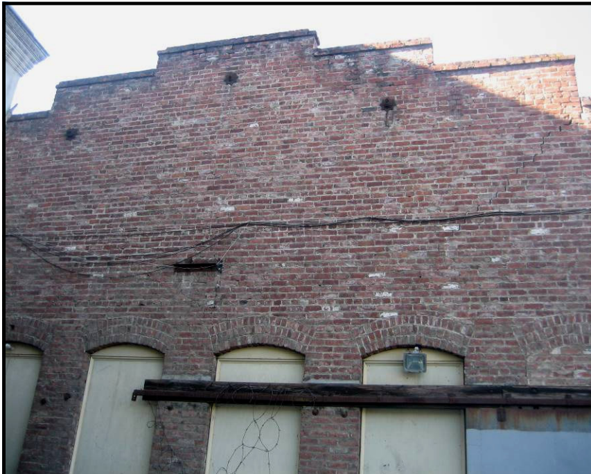
Top, back wall of Letcher's second garage on the No. First & St. James Streets. Note the steel shutters. Above, back wall of Letcher's third garage at 214 North First street, right next door.
